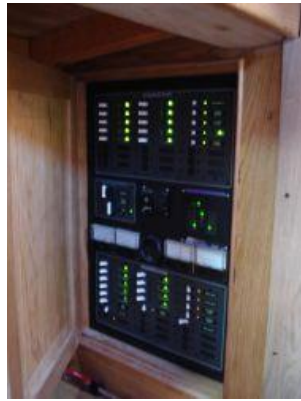
New & Hidden Elec. Service Panel
