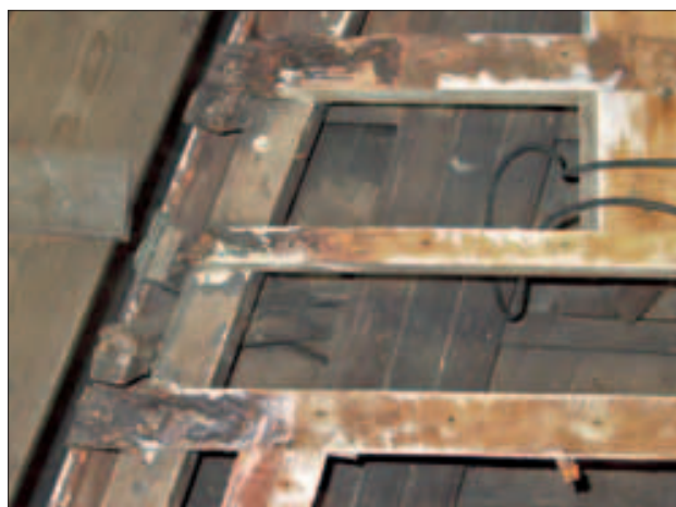
Decayed frame ends
